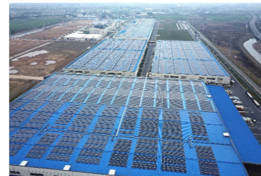
Installation Site: Changzhou Base Size of the System 14.45MW
