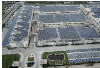
Installation Site: Ninghai Base Size of the System 3.7MW
